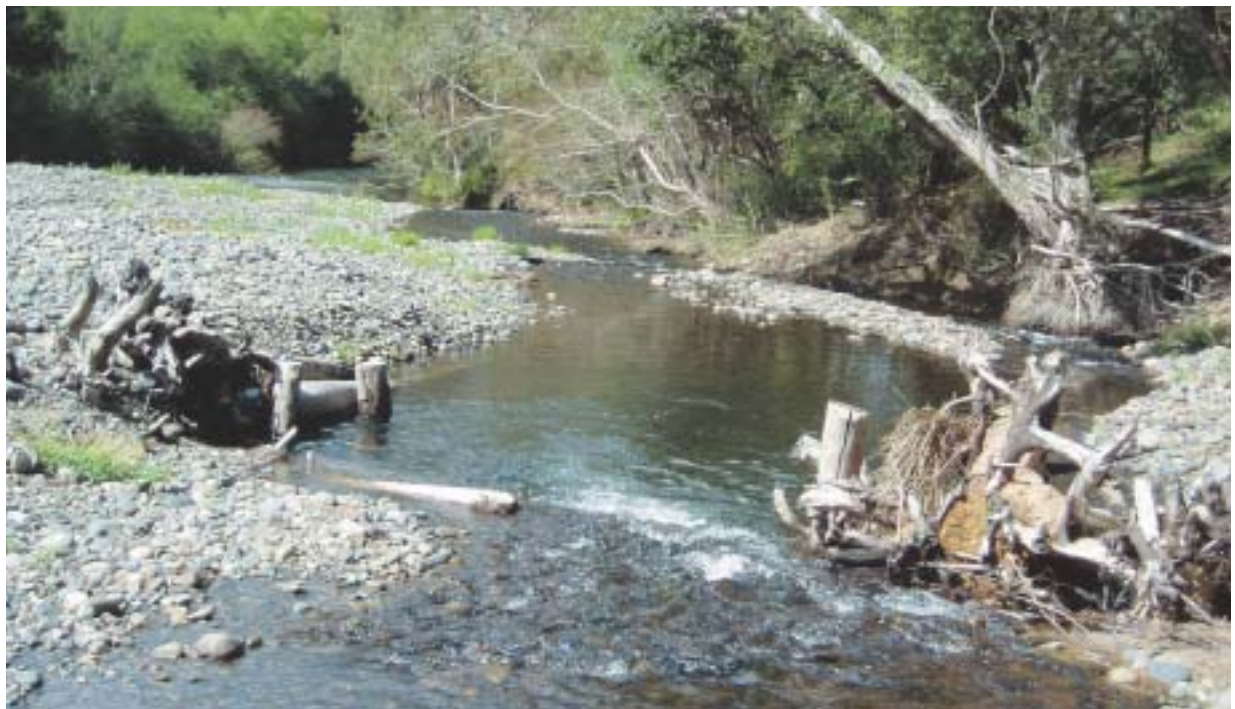
Photo 7 (below). Constructed hyporheic jam (i.e. log step with paired abutment jams) — Williams River, NSW.
